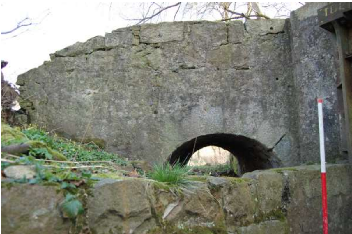
Illus 60 Earlier lade S15 blocked by north wall lade S6; facing ENE
