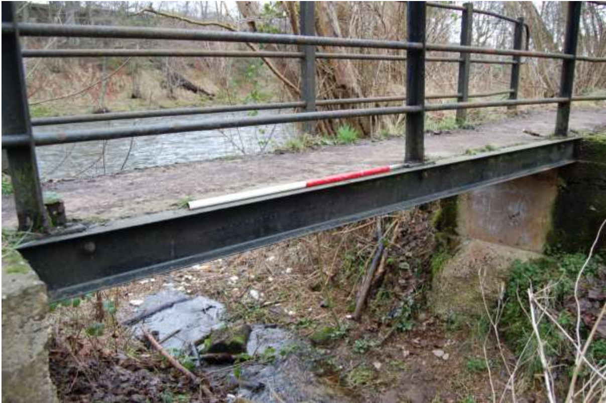
Illus 93 Bridge S28 with steel beam marked 'LANARKSHIRE STEEL CO LTD SCOTLAND 7 x 4' with 'BRITISH STEEL'
