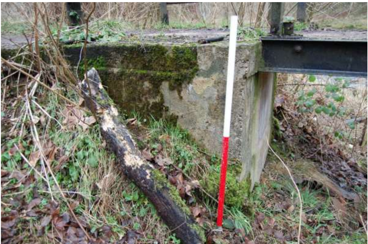
Illus 92 Bridge S20 poured concrete pier on the west side of the bridge
