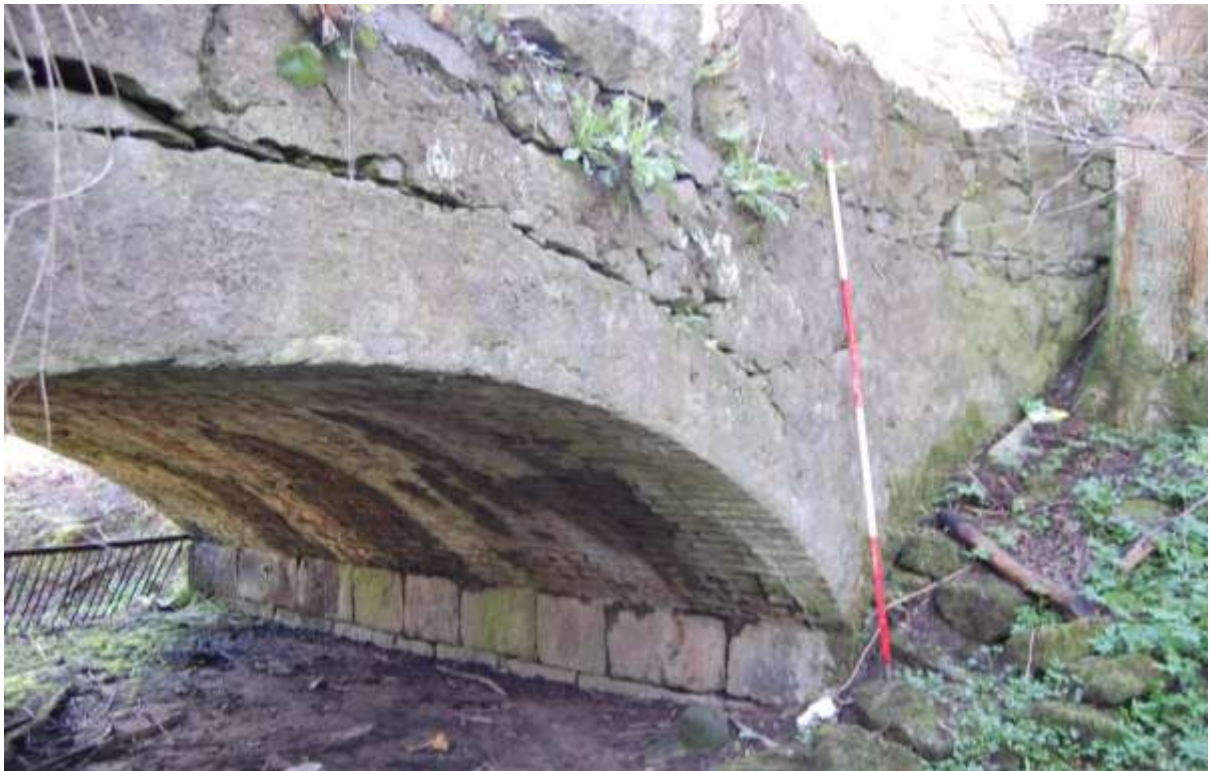
Illus 99 South face and east pier of culvert S33 with bridge above showing brick vaulting on stone foundation; facing E
