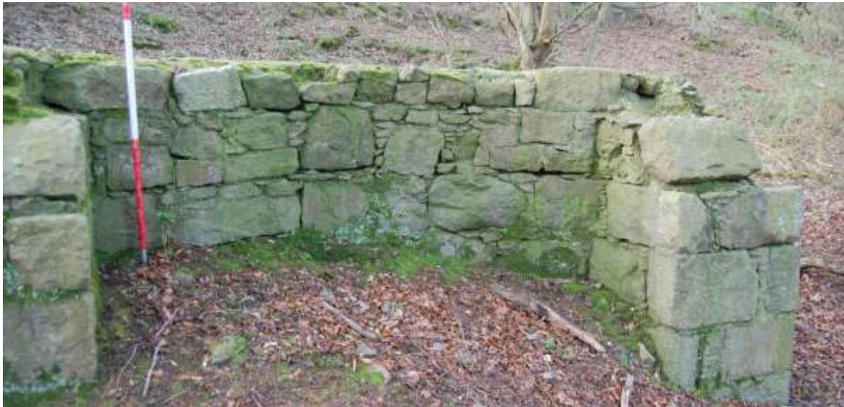
Illus 4 Structure 1 showing sections of convex curving wall between buttresses; facing S
