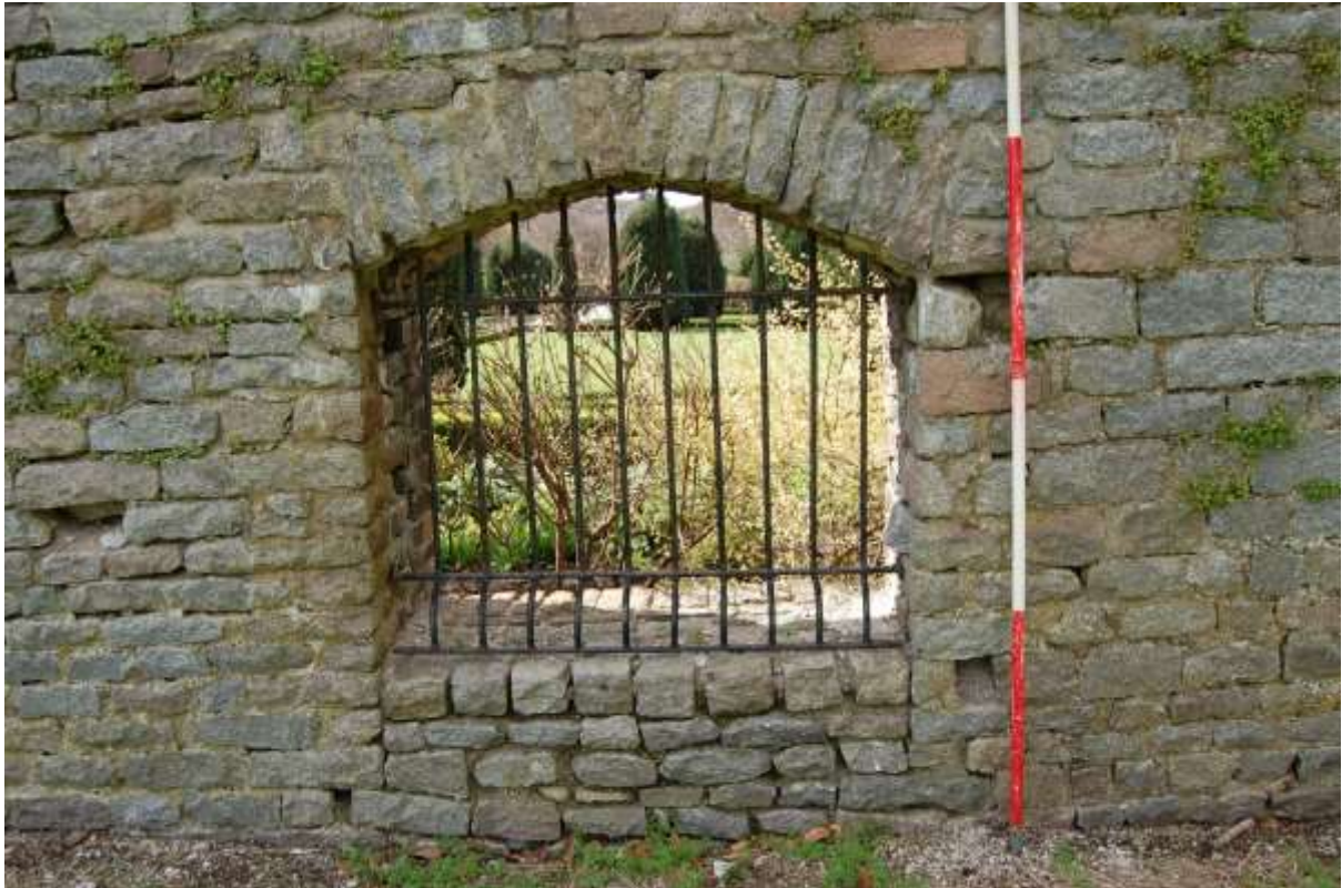
Illus 79 Former door converted to window in centre of east wall; facing W
