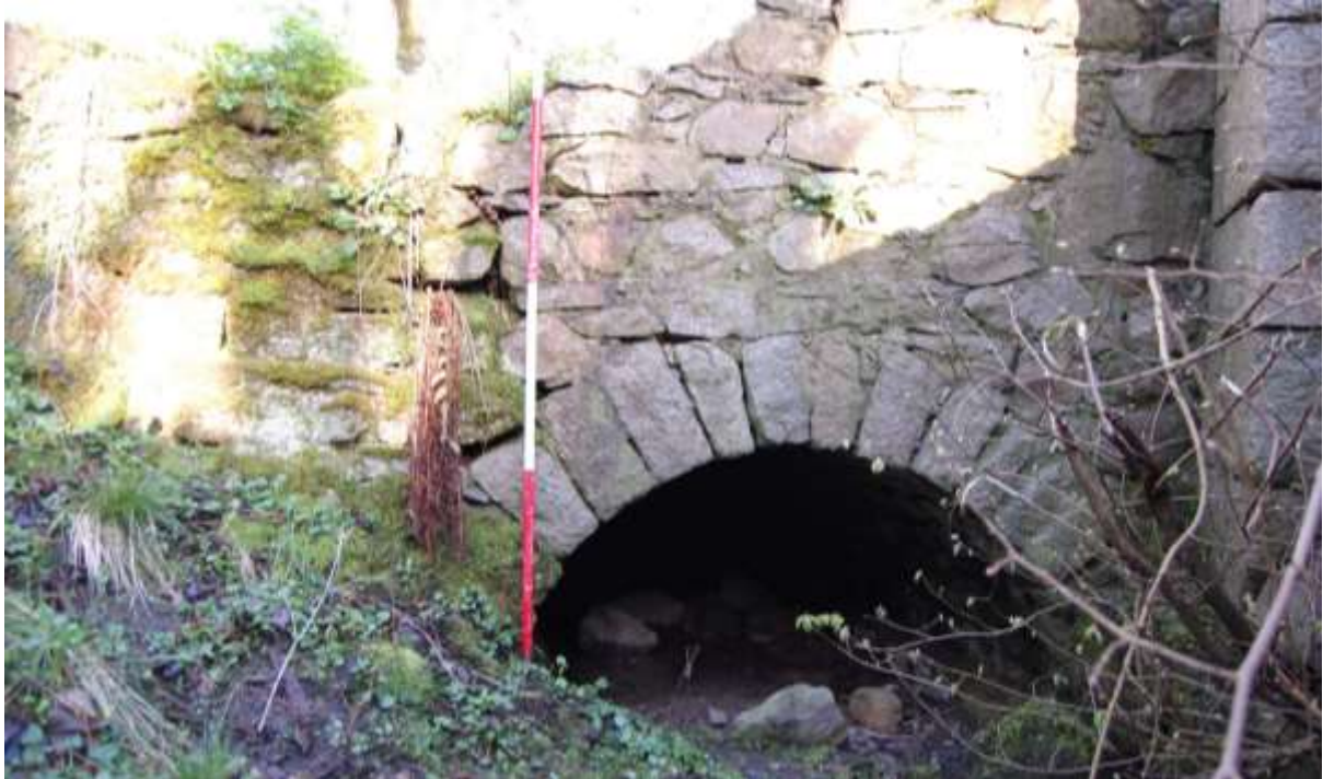
Illus 104 Culvert S36 showing stone vaulting with bridge and culvert S33 (right); facing NW
