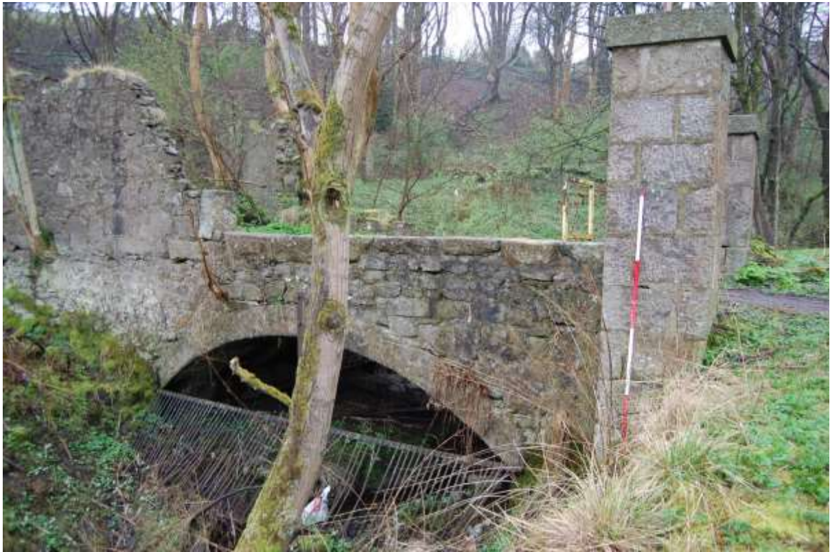
Illus 98 North face of culvert and bridge S33 for lade S13; facing SSW
