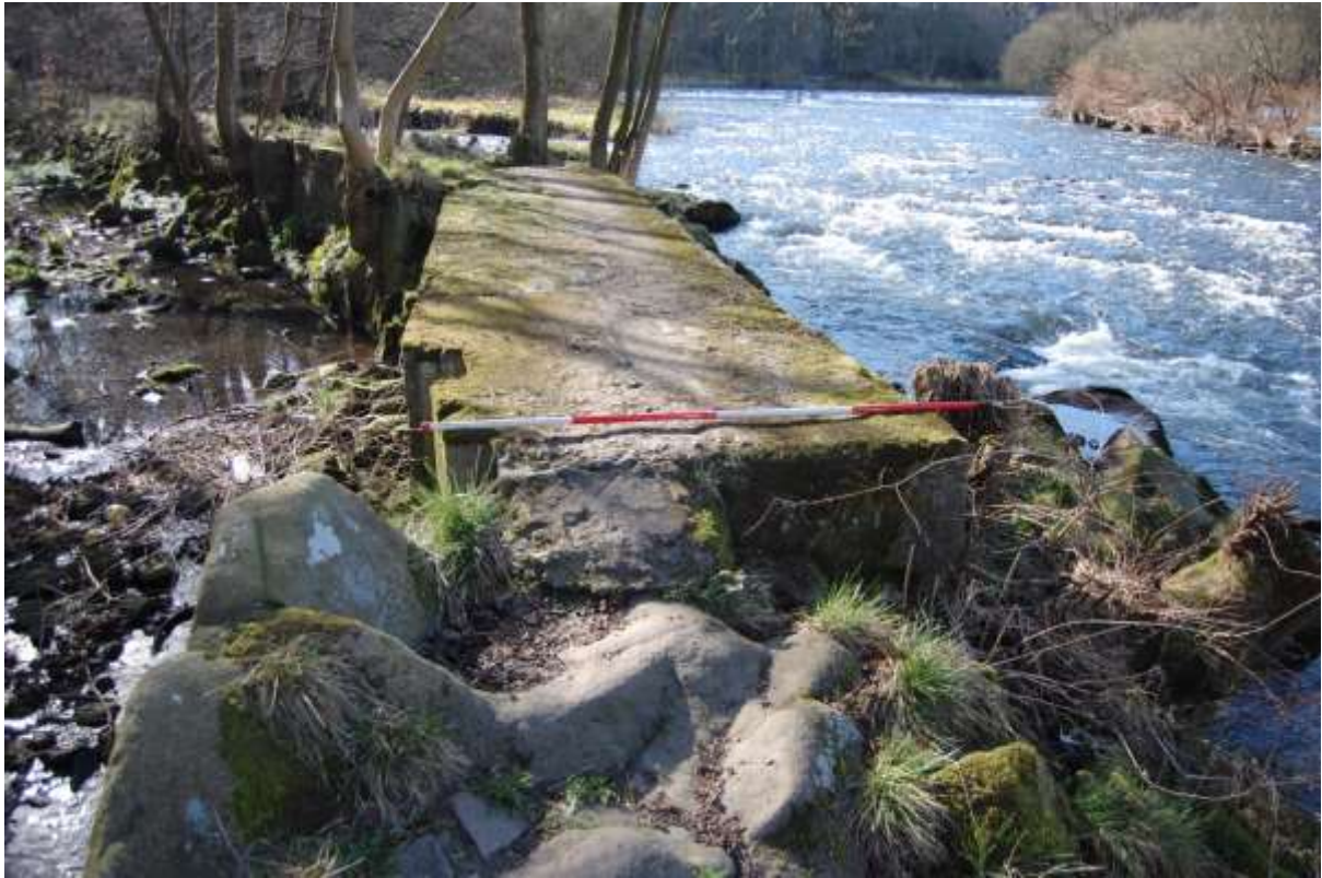
Illus 85 Remains of sluice S26 with river Don (right) and lade S6 (left); facing S
