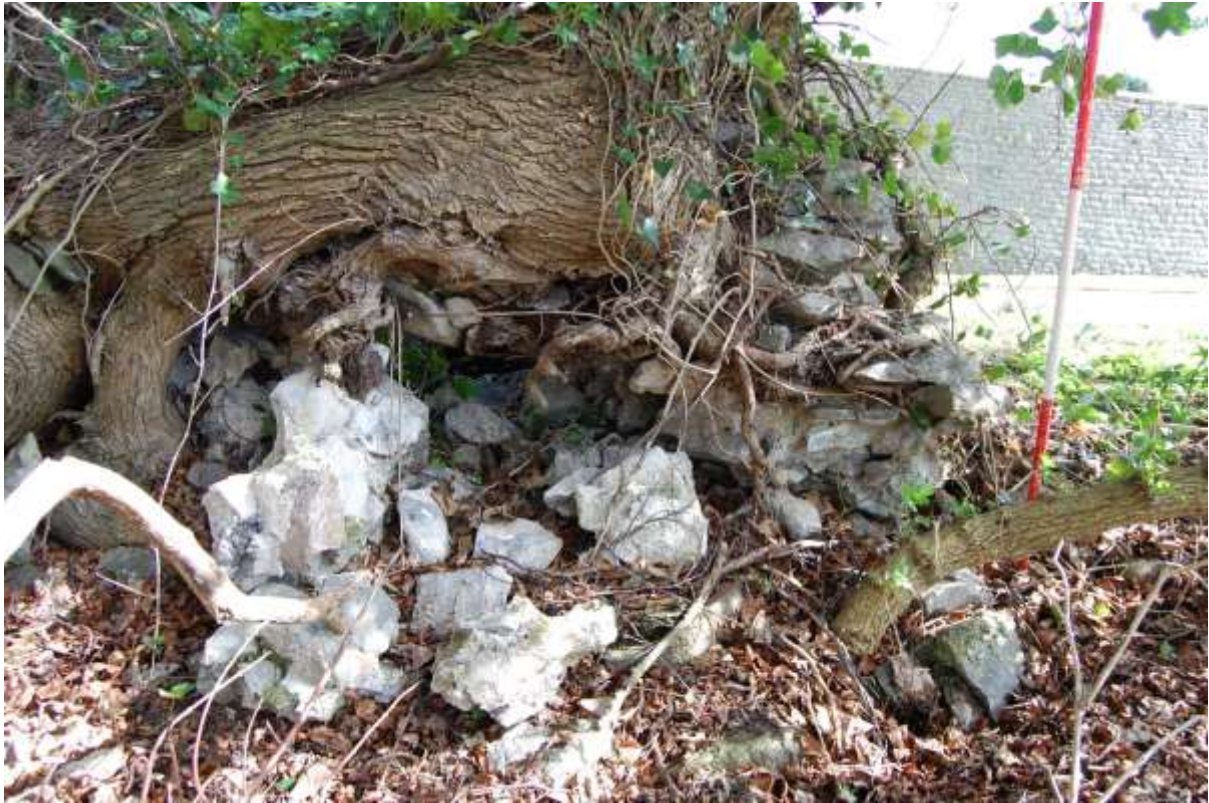
Illus 108 Rear (west side) of structure 37 showing damage due to tree virtually obscuring the feature
