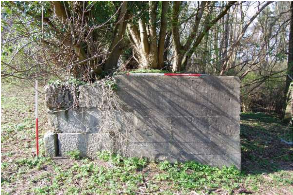
Illus 23 East end lade S6 wall showing stone structure (left) with poured concrete extension (right); facing W
