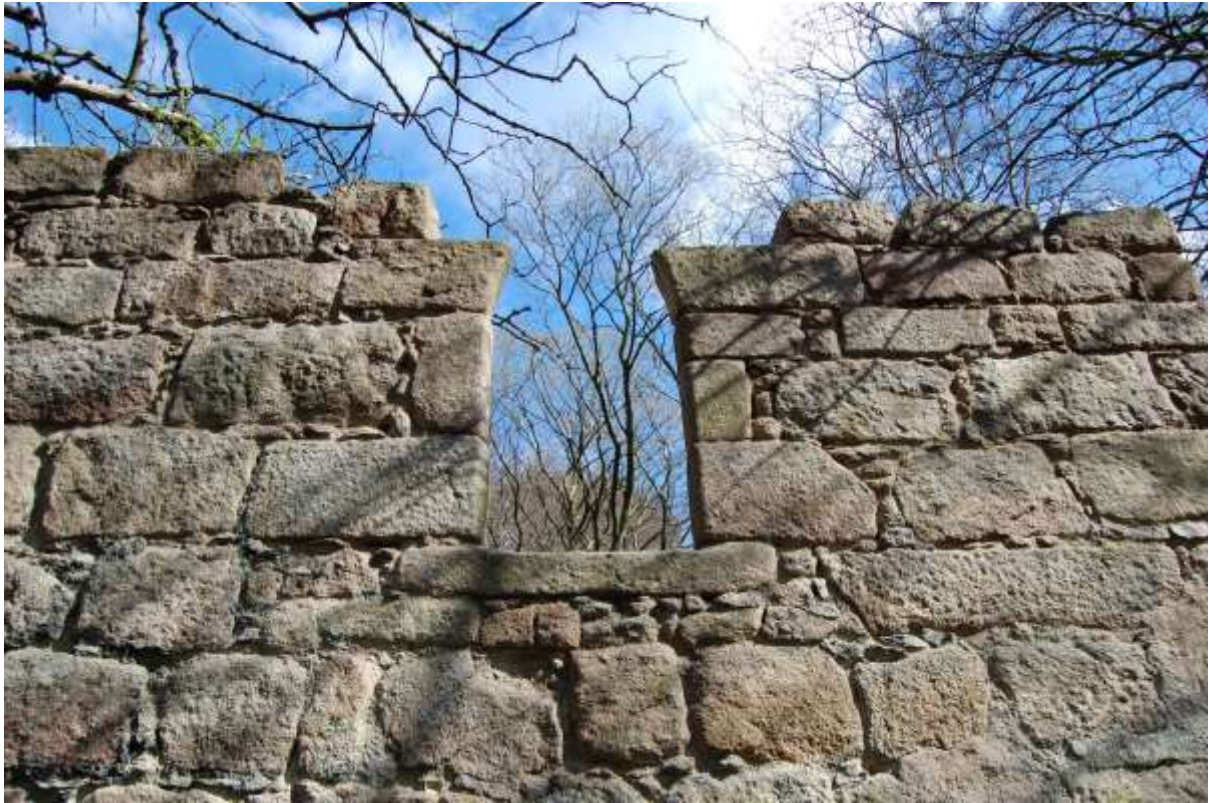
Illus 66 Structure 16 West wall showing arched window formed using granite blocks; facing E
