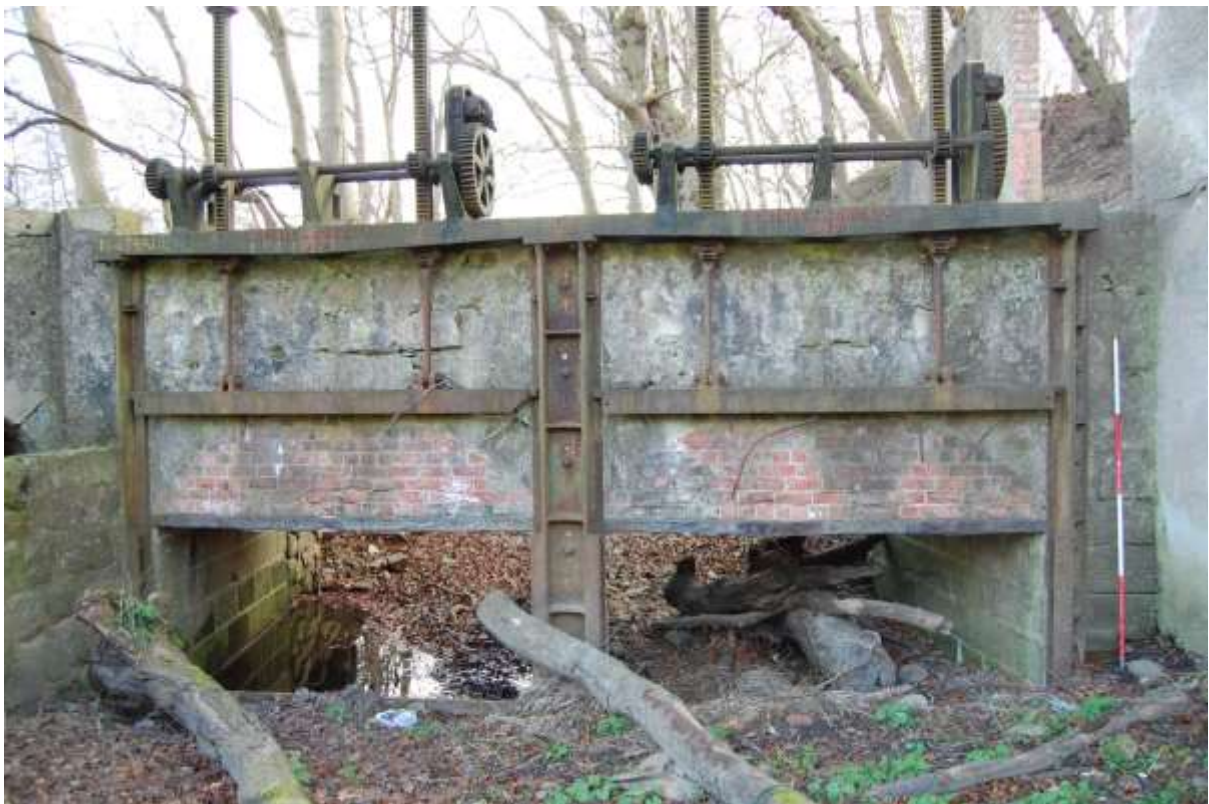
Illus 55 Sluice gate structure on the west side of the bridge marked 'A Pirie & Sons 1919'.
