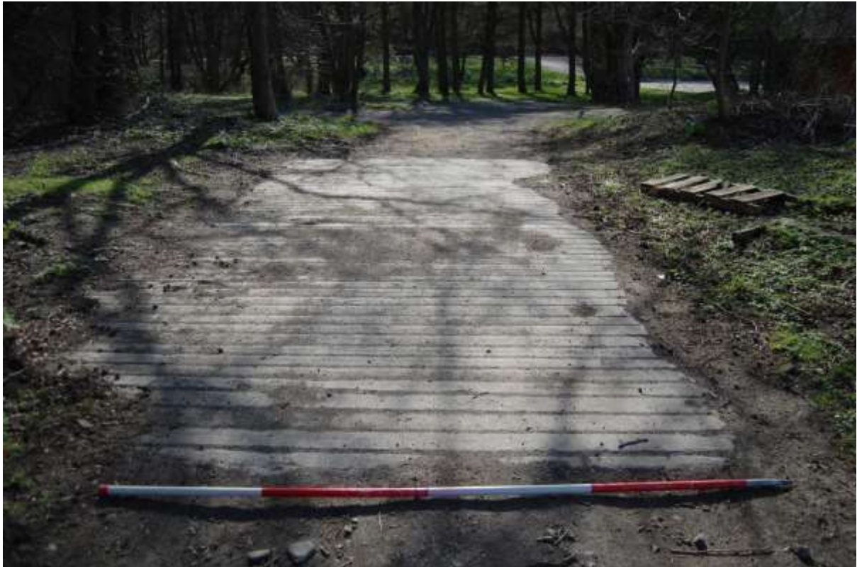
Illus 82 Poured concrete bridge taking footpath over remains of Lade 6; facing NNE
