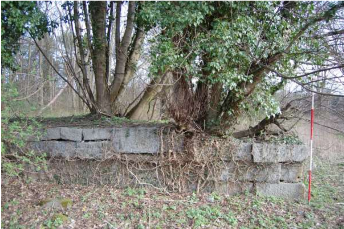
Illus 20 Facing of north wall of lade S6 at east end showing damage due to established trees; the line of the lade ran long the foreground of the photograph but has been completely infilled
