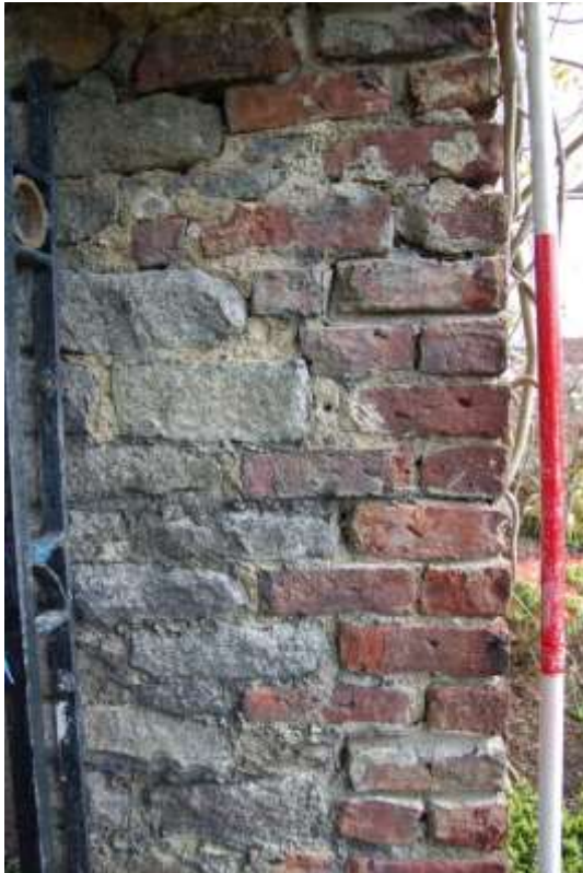
Illus 77 Section of north wall walled garden S19 showing interior (right) lined with brick; facing E
