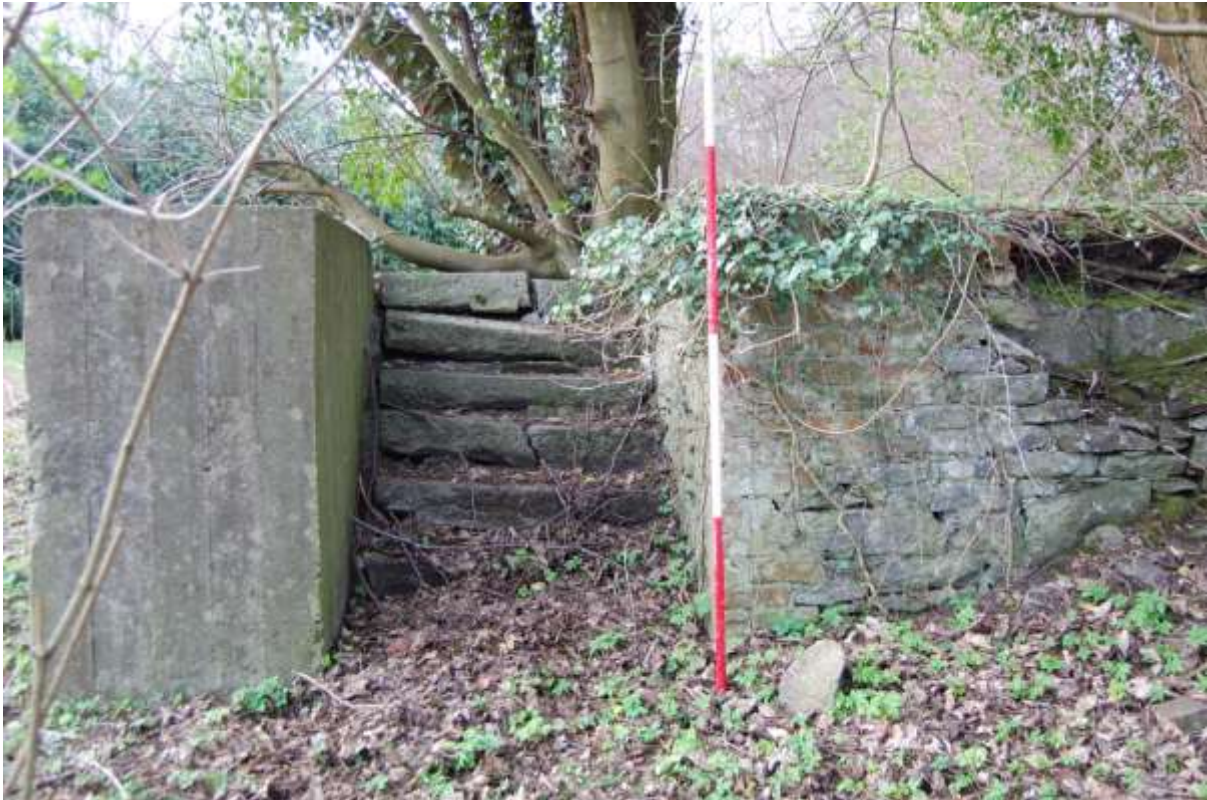
Illus 24 East end lade S6 wall showing stone steps and stone and brick structure (right) with poured concrete extension (left); facing W
