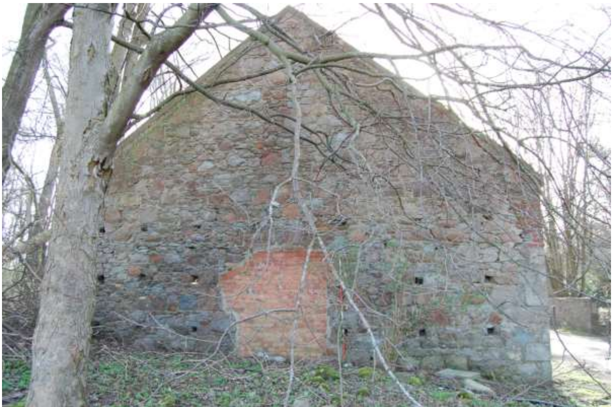
Illus 12 West gable of Structure 3, originally an interior wall prior to demolition of west end of building; facing E
