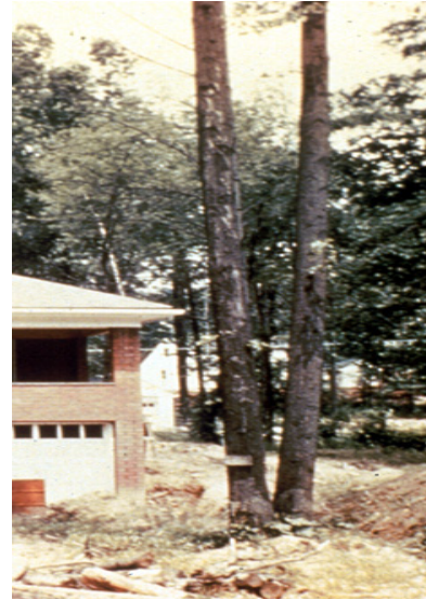
Figure 1 - Soil fill around tree. Note lack of flare at base of trunk.
