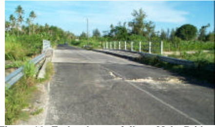
Figure 13: Embankment failure, Mele Bridge
