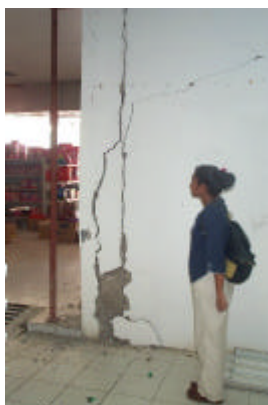
Figure 6: Damage around ground-floor columns at Au Bon Marche
