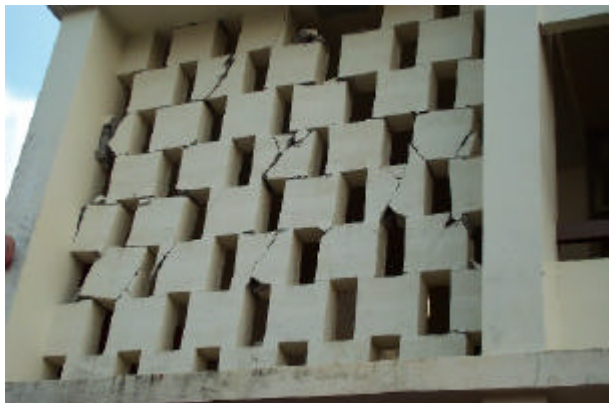
Figure 5: Infill blockwork in stairwells sheared and collapsed
