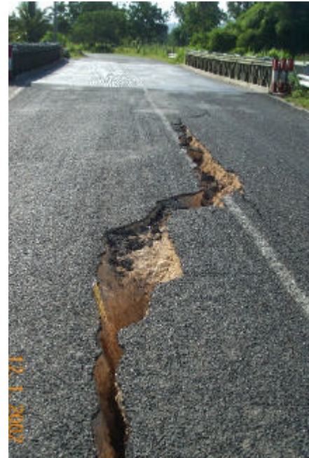
Figure 15: Embankment failure, Prima Bridge
