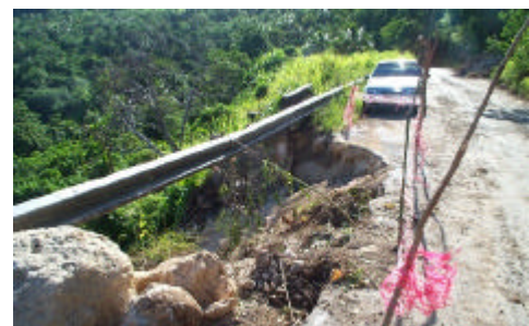
Figure 20: Road embankment collapse, Klem's Hill
