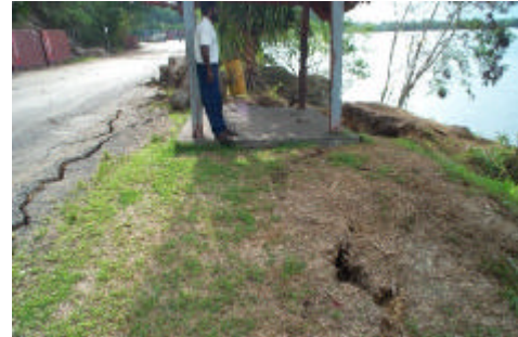
Figure 18: Road embankment collapse, Wharf road
