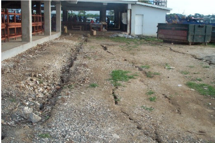
Figure 7: Fissuring in back-fill behind sea wall, north of Market
