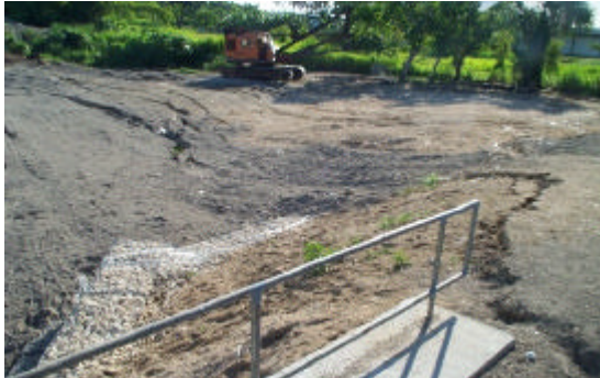
Figure 14: Slumping due to liquefaction, Prima Bridge
