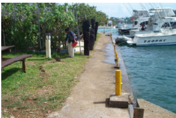
Figure 10: Ground fissures and tilted sea wall near Waterfront Bar
