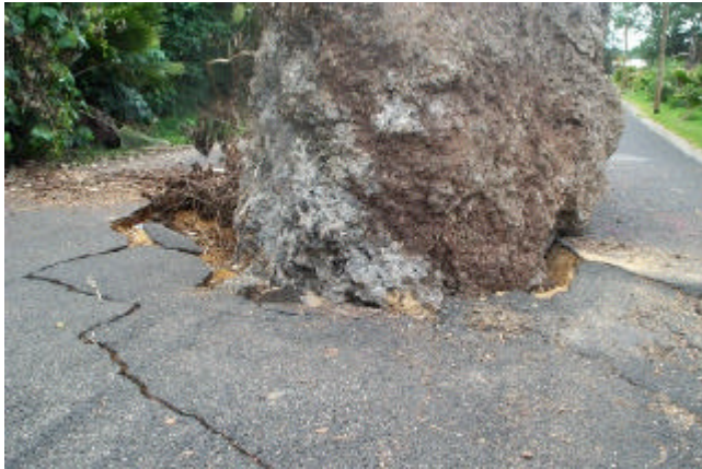
Figure 17: Toppled limestone boulder puncturing road surface
