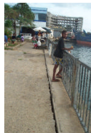
Figure 11: Gap between sea wall and back-fill
